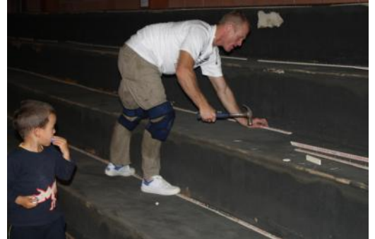
Hard at work... David Longhurst (and son) laying the new carpet . And pictured left the finished result....da da !
